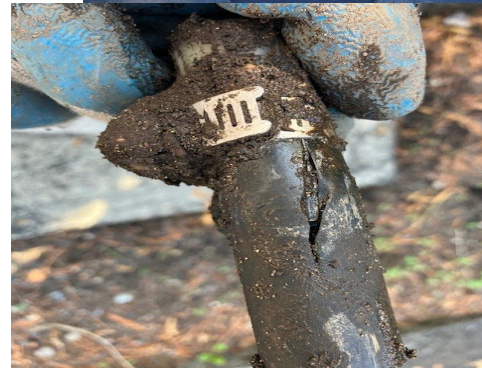
1970's Era Polyethylene Water Service Leak
